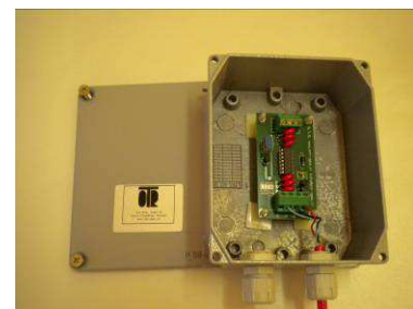
4-20 mA transmitter (Code O00LCE00420 ) Inside a Junction box
