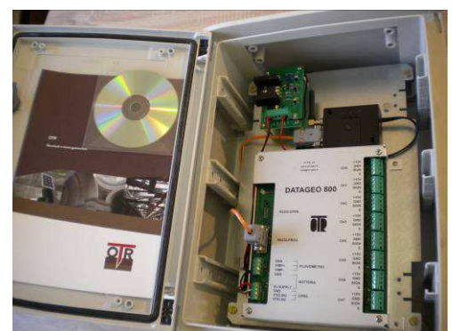
Data acquisition system datalogger D800 (Code O0D800C0008)
