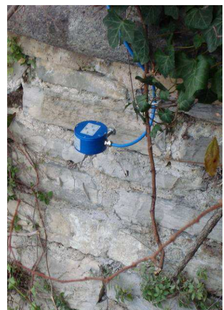
Biaxial tiltmeter on the wall
