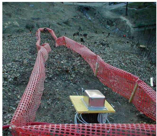
Wire extensometer installation in landslide
